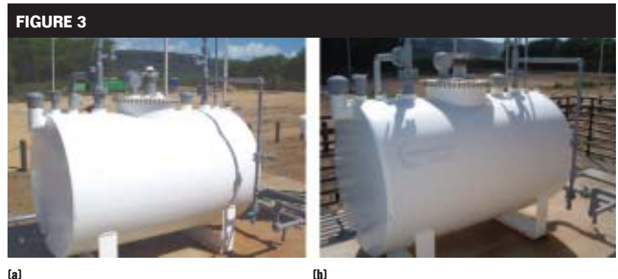
West side (ocean side) of storage tank at block house with appliqué. (a) September 2004—appliqué as installed, and (b) October 2005.
