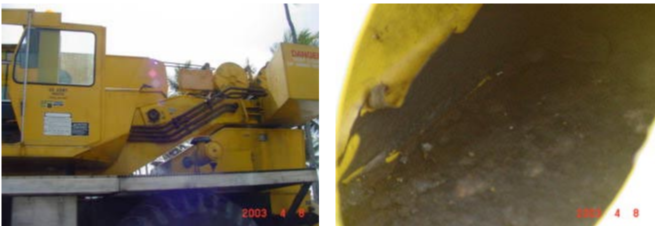
Figure 2. Left: Boom truck on Kwajalein Atoll. Right: Close up of corrosion that made boom truck unsafe and inoperative after only 3 years.
